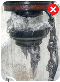
Plugged Submersible Pumps
